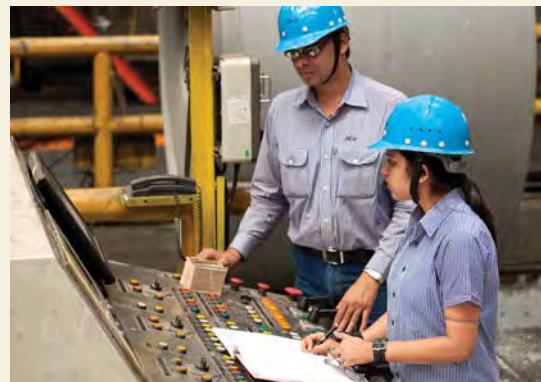
Employees at the Control panel of the CRM Complex
